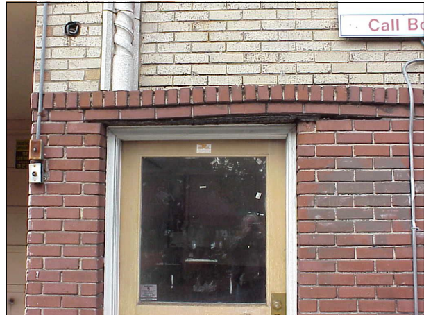
Oxide Jacking at steel lintel
