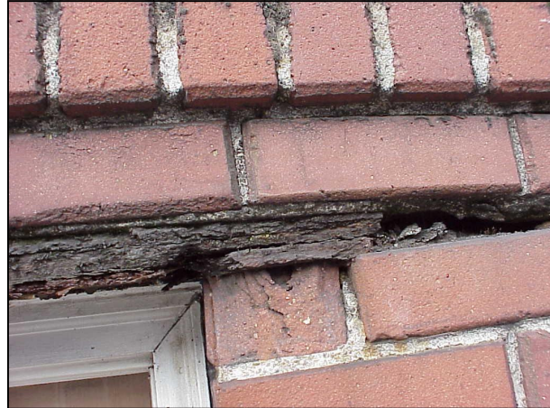
Oxide growth at unrestrained side of steel lintel is much greater than loaded side
