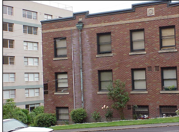
Water damage from leaking scupper (above)
