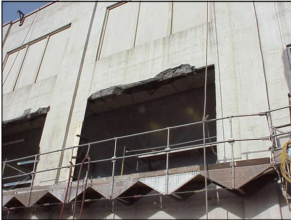
Spalling Concrete at Window Headers Poorly Consolidated Concrete
