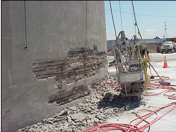
Glacier Northwest Silo 14 Spalling Concrete at Base After Removal of Loose Concrete
