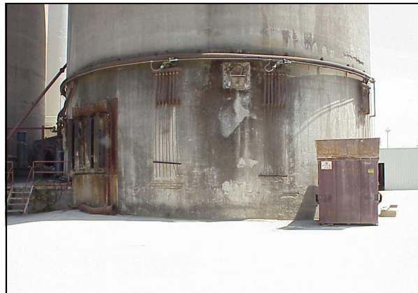
Glacier Northwest Silo 14 Spalling Concrete at Base Prior to Removal of Loose Concrete
