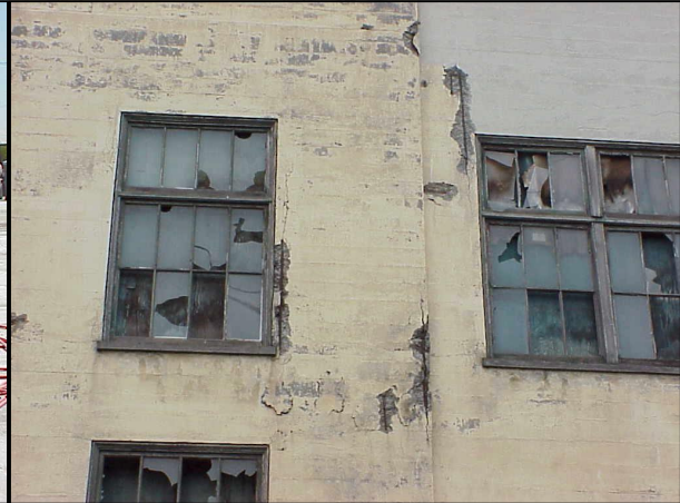
Pacific Coast Feather Typical Concrete Spalling at Window Jambs, Field and Corners
